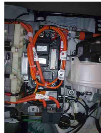
Figure 4 HV battery view
