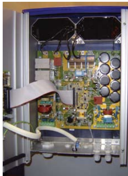
Figure 7: Small inverter for 3kWp output power
